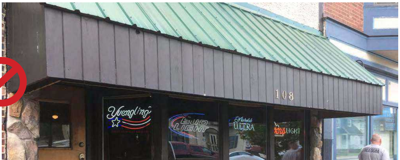
Do not build structured awnings that cover up historic storefront details such as transoms, columns, or cornices.
