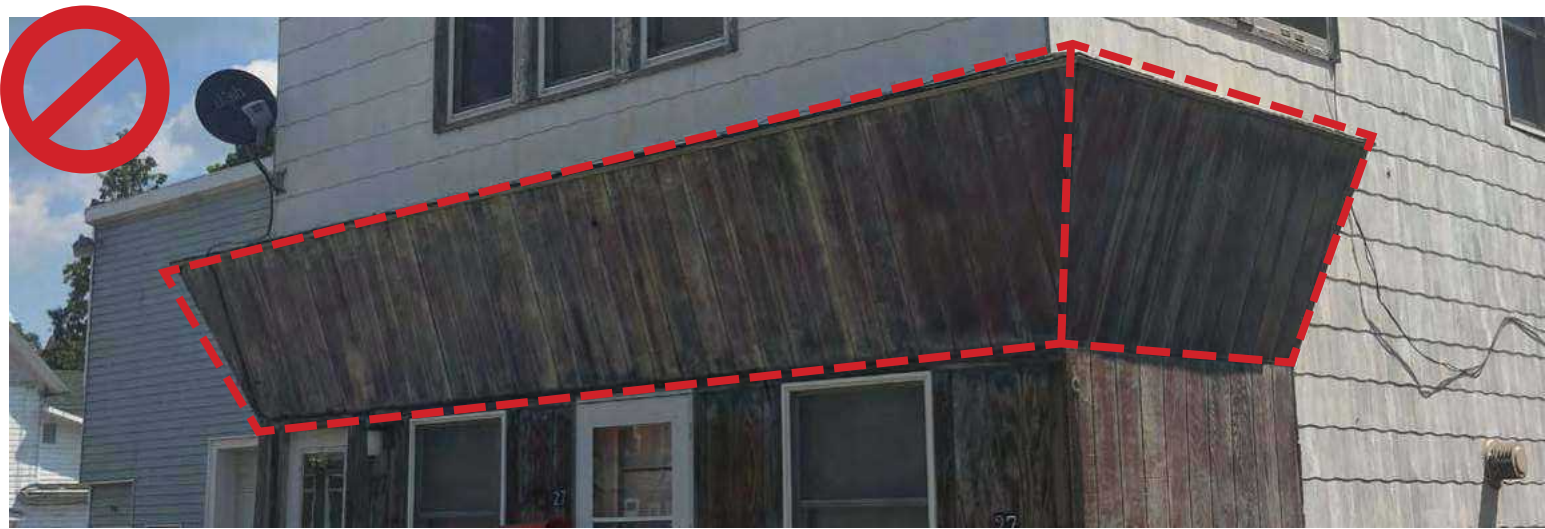
Avoid covering up original storefront elements, such as cornices, signboards, or transom windows.
