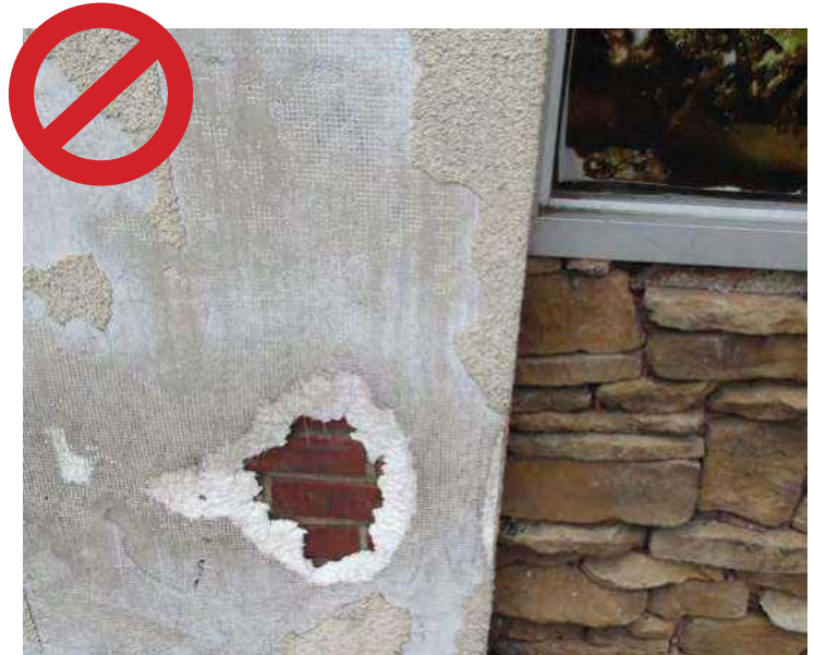
Do not use EIFS to cover original materials or in places requiring increased durability.
