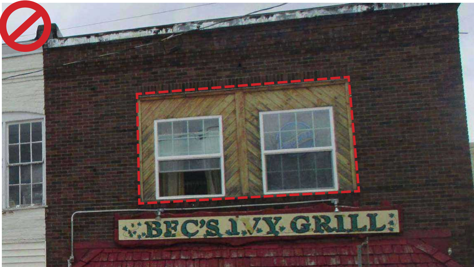
Do not fill in large upper floor window openings with smaller, undersized vinyl windows.
