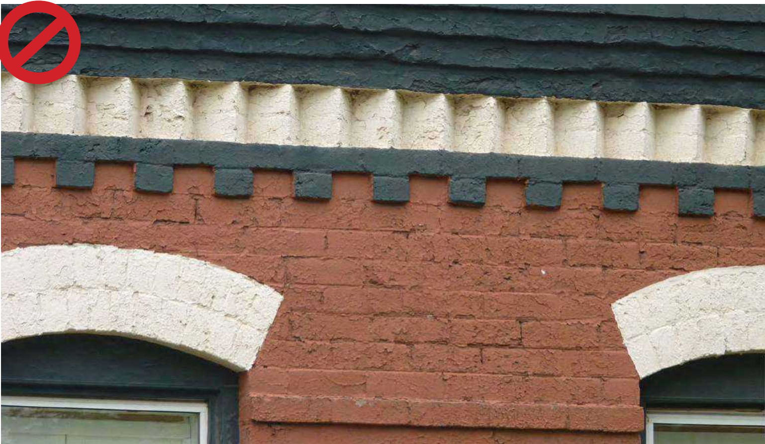
Repair aged masonry surfaces before repainting to avoid flaking paint with a reduced lifespan.
